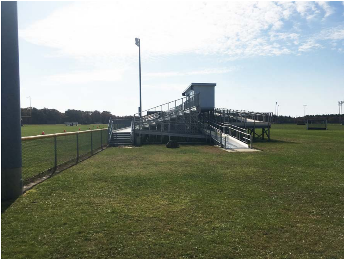
Figure 8 – Access to grandstands is not ADA compliant.
